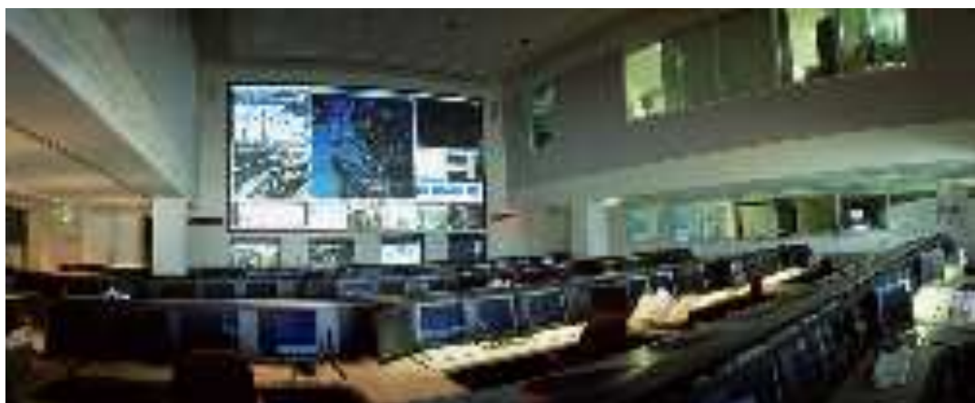
California Dept. of Transportation (Caltrans)
